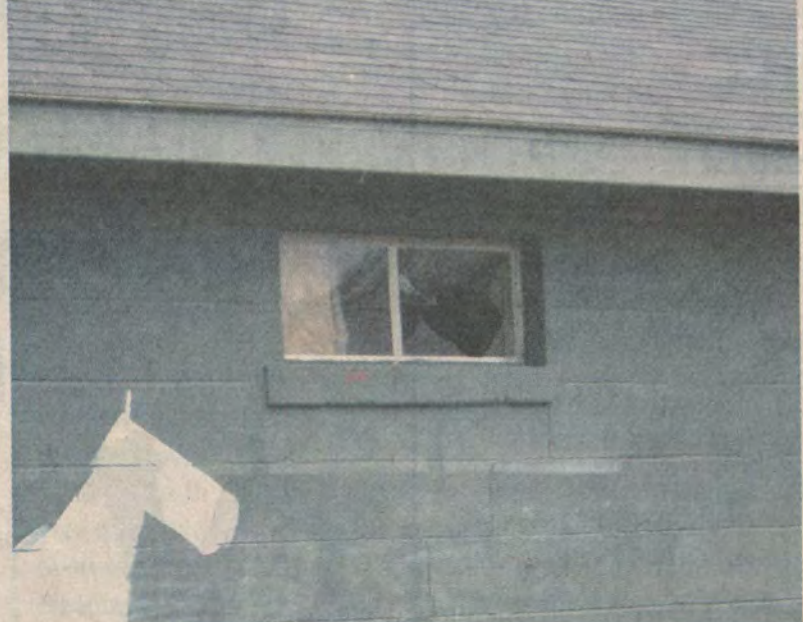
A broken window is but one of several damages sustained by the MOBROC barn. (Solod)
