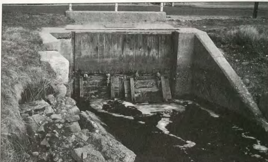
Fig.2 A pair of tidal gates on Sybil Creek, Branford (R. Rozsa)
