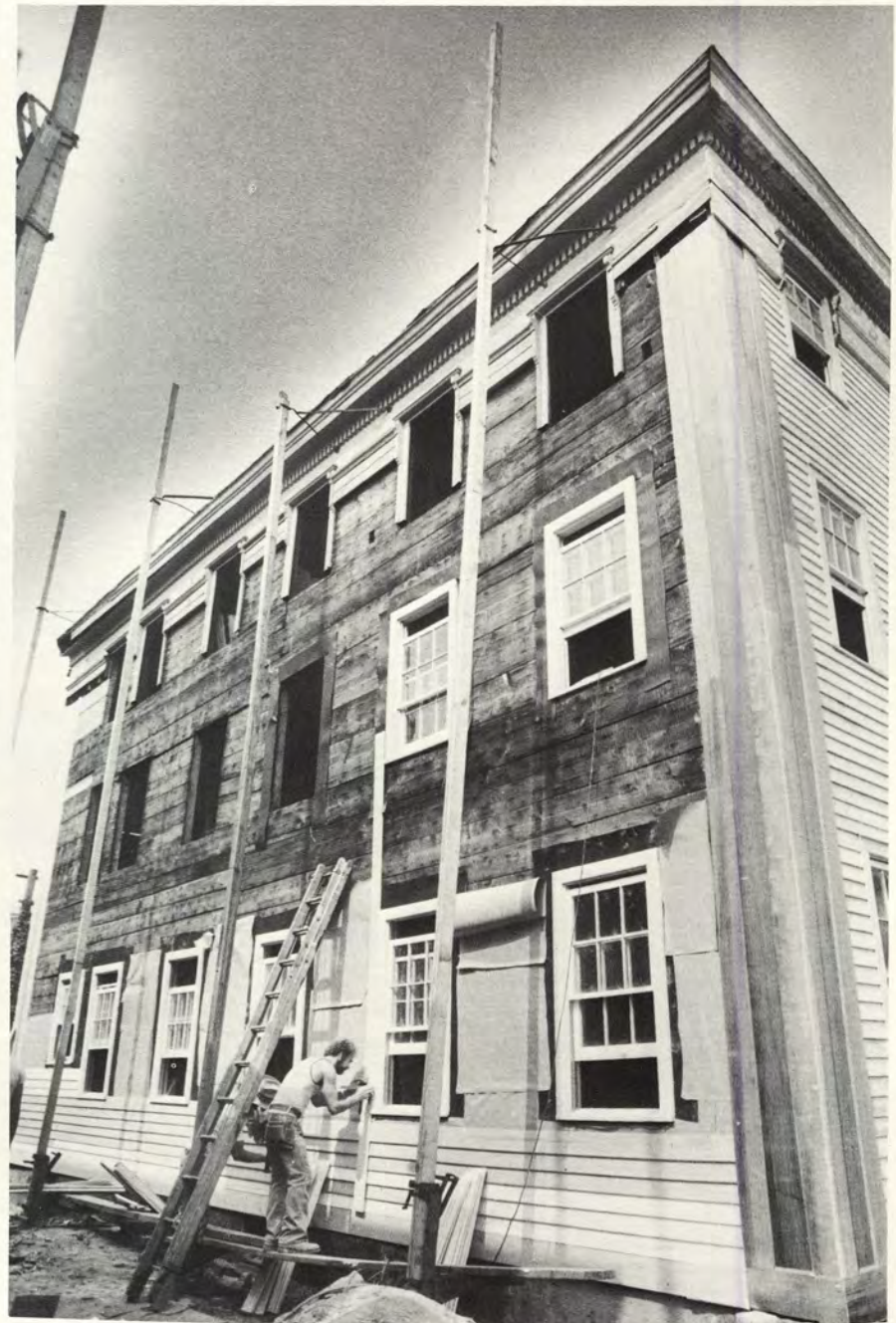
New clapboards are going up on the magnificent No. 16 Starr Street (right).
