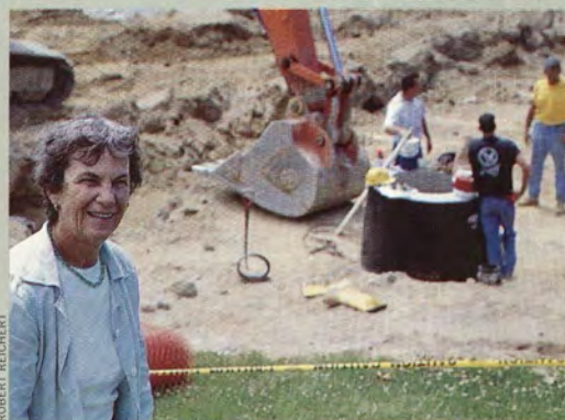
VIRGINIA SLAUGHTER LOEB '48 P'77, CONNECTICUT COLLEGE TRUSTEE AND MOTHER OF TOM SLAUGHTER '77, SURVEYS THE CONSTRUCTION PROGRESS.
