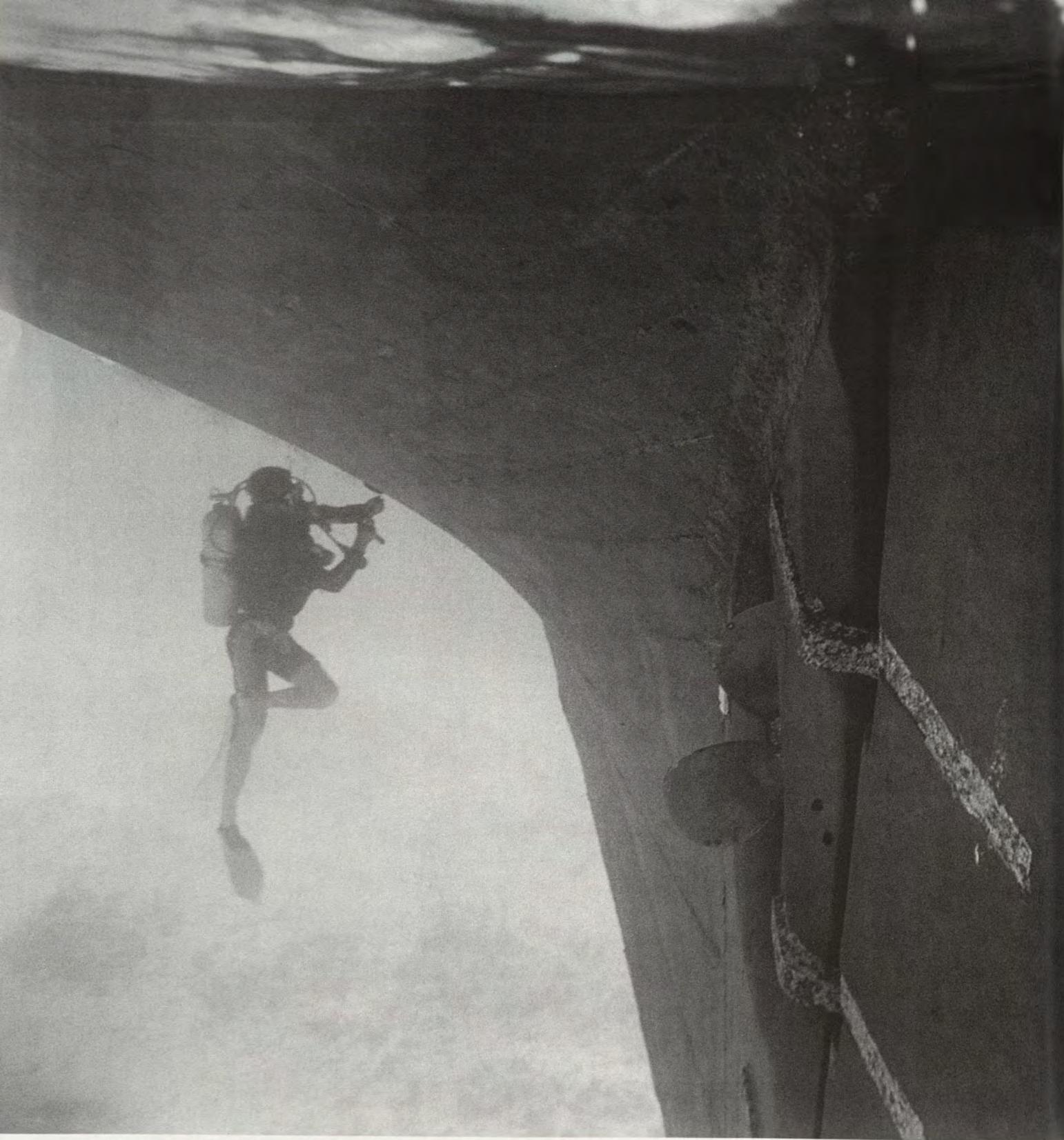
CAPTAIN CHRIS MCGUIRE '93 MAKES SOME HULL REPAIRS AT ANCHOR IN THE BAHAMAS.
