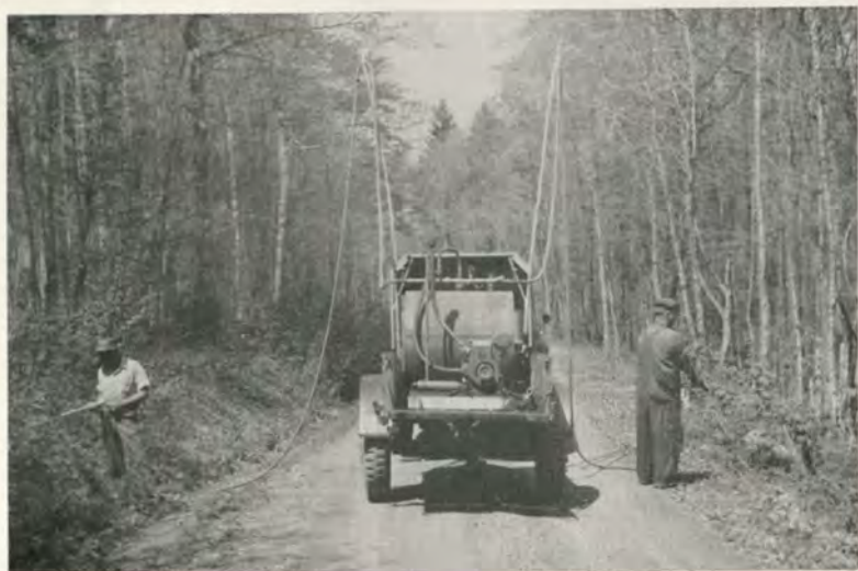
Fig. 2. A power sprayer, converted from a standard model fire-control pumper, in use on a road on the Monongabela National Forest. The poles hold surplus hose off the ground and out of the way when spraying close to the truck, as shown here. When the full length of hose is needed, it is readily available.
