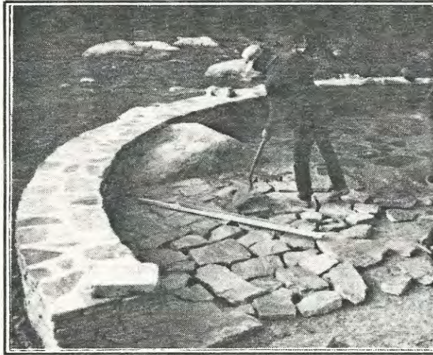
Mason Mark Gleason installs the patio adjacent to the dwarf conifer display in the Gries Memorial Native Conifer Collection. Fall, 1988.
