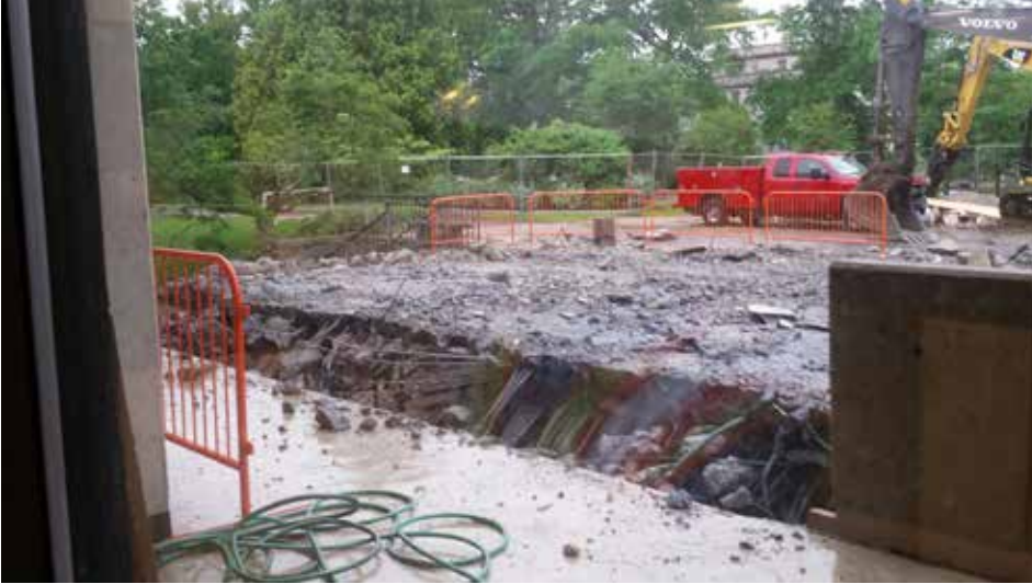
IN PREPARATION FOR BUILDING THE NEW ENTRANCE AND PATIO, CREWS FIRST DEMOLISHED THE BRIDGE OVER THE LIBRARY'S MOAT.
