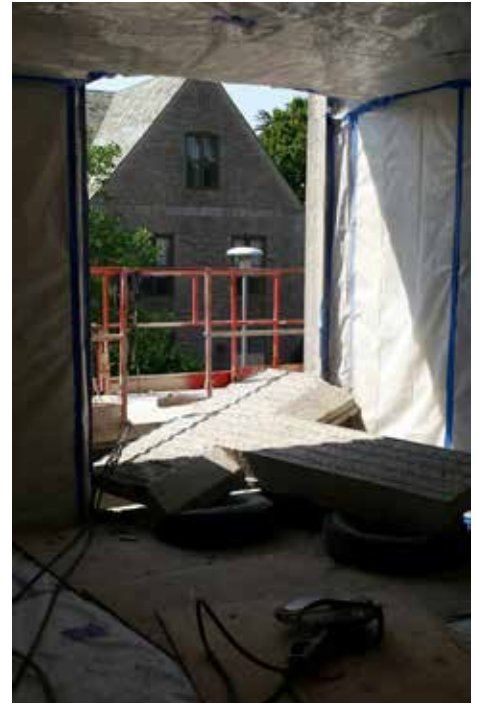
THIS PHOTO OFFERS A PEEK THROUGH THE FIRST ENLARGED WINDOW THAT WAS CUT, WITH A VIEW TOWARD BLAUSTEIN HUMANITIES CENTER. NUMEROUS WINDOWS ON THE SOUTH, EAST AND NORTH SIDES OF THE BUILDING WILL BE ENLARGED TO PROVIDE ADDITIONAL LIGHT.
