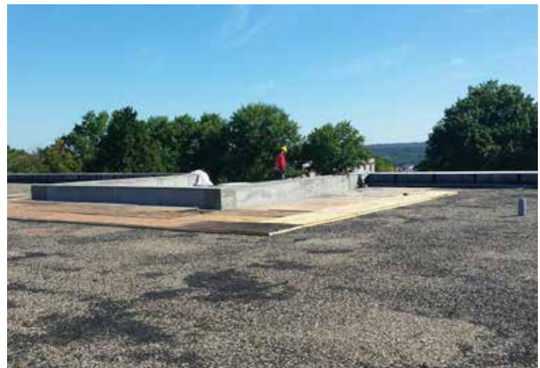
WORKERS PREPARE THE LIBRARY'S ROOF FOR THE PLACEMENT OF THE "MONITOR," THE STRUCTURE THAT WILL EXTEND FROM THE ROOF TO ENCASE A NEW GLASS FAÇADE
