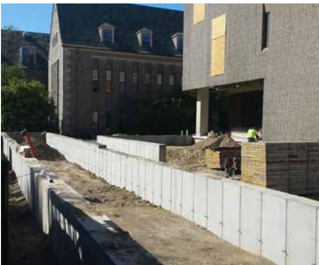
BY EARLY SEPTEMBER, THE FRONT PATIO AND PLANTER HAD BEGUN TO TAKE SHAPE.
