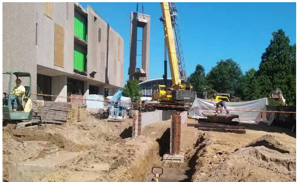
THE SHAIN LIBRARY RENOVATION TOOK A BIG STEP FORWARD ON AUG. 19, WHEN LARGE SECTIONS OF CONCRETE WERE REMOVED TO MAKE WAY FOR A GLASS ENCLOSURE.
