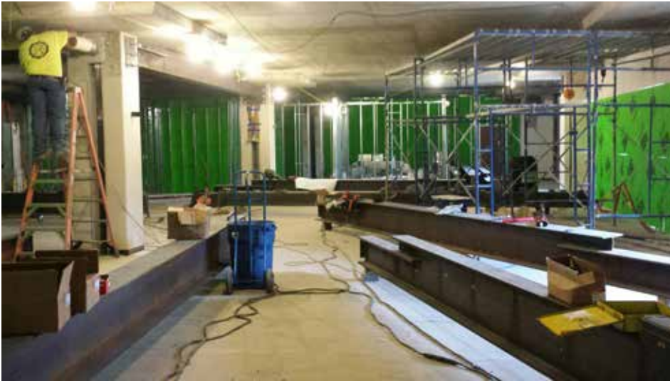
CREWS BEGIN TO PLACE THE STEEL IN WHAT WILL BECOME THE THIRD-FLOOR READING ROOM.
