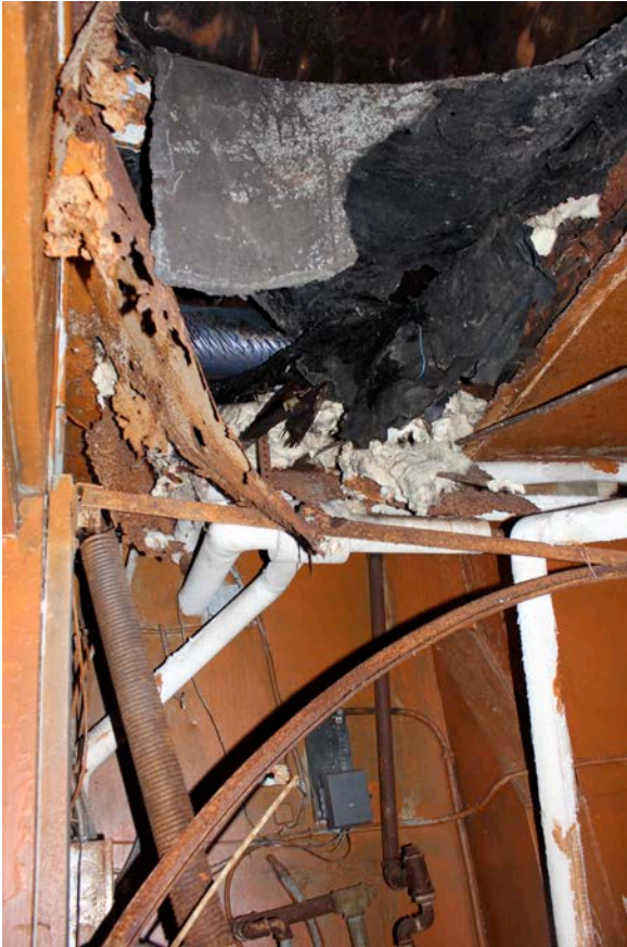
Damage to the garage roof
