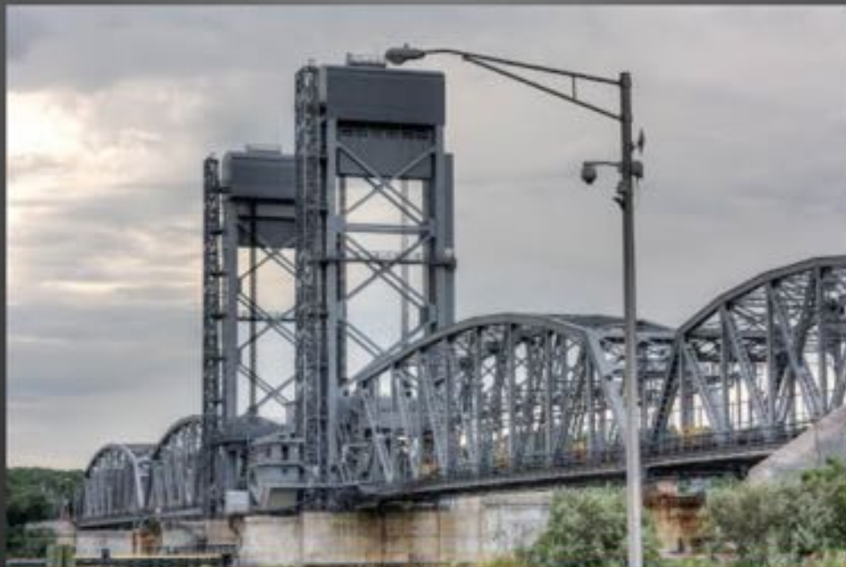
Thames River Bridge (Amtrak), New London and Groton, CT, originally a 1919 Warren through truss bascule design, changed to a lift bridge in 2008
