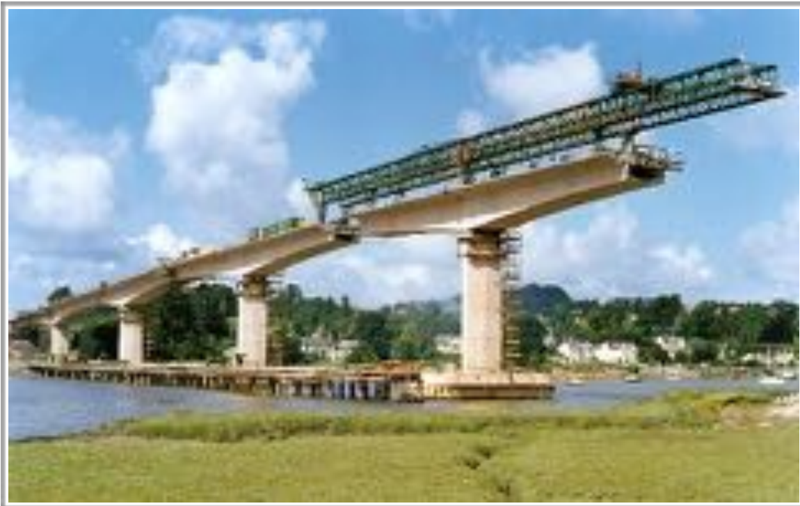
Figure 9.1: Example of a reinforced concrete box girder being lowered into place on a construction site
