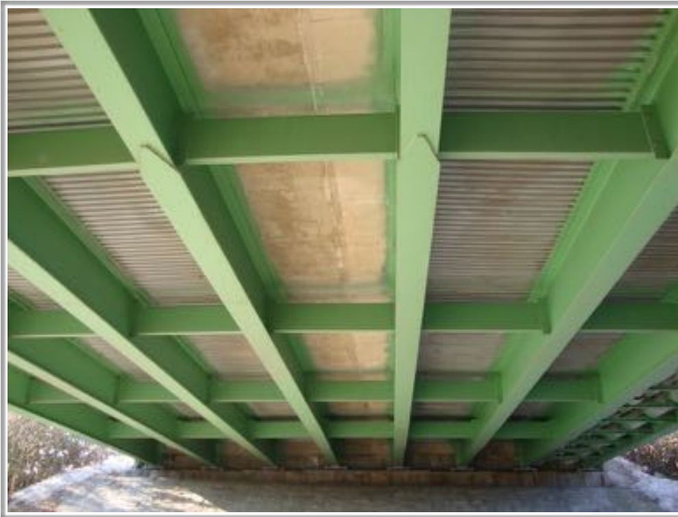
Figures 10.1, 10.2, 10.3: Example of a finished metal rolled multi-beam bridge and images showing the metal rolling process
